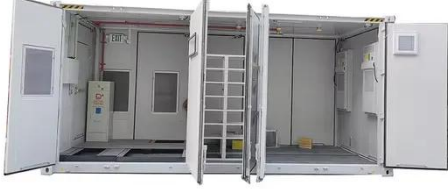
1075KW HH ESS
