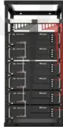
Cabinet and rack installation display
